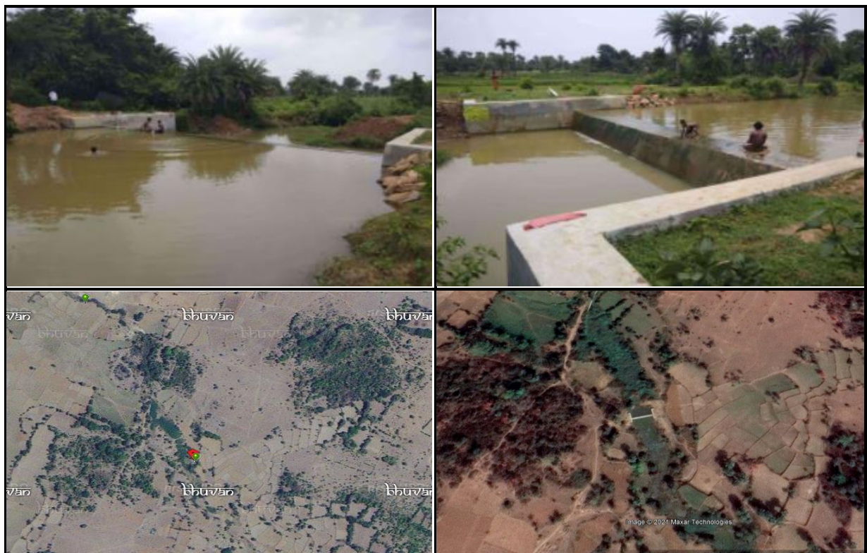
Figure 3-24 Cemented Check Dam, Lathibari Village (a) Geotagged Photographs (b) NABARD Bhuvan Portal (c) Google Earth of Lathibari watershed
